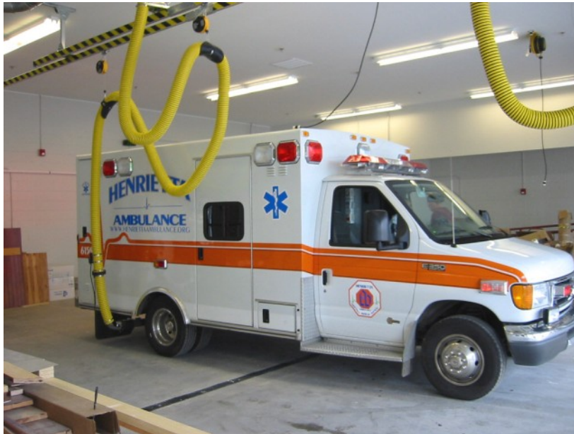
6159, our newest ambulance attached to the Plymovent System
